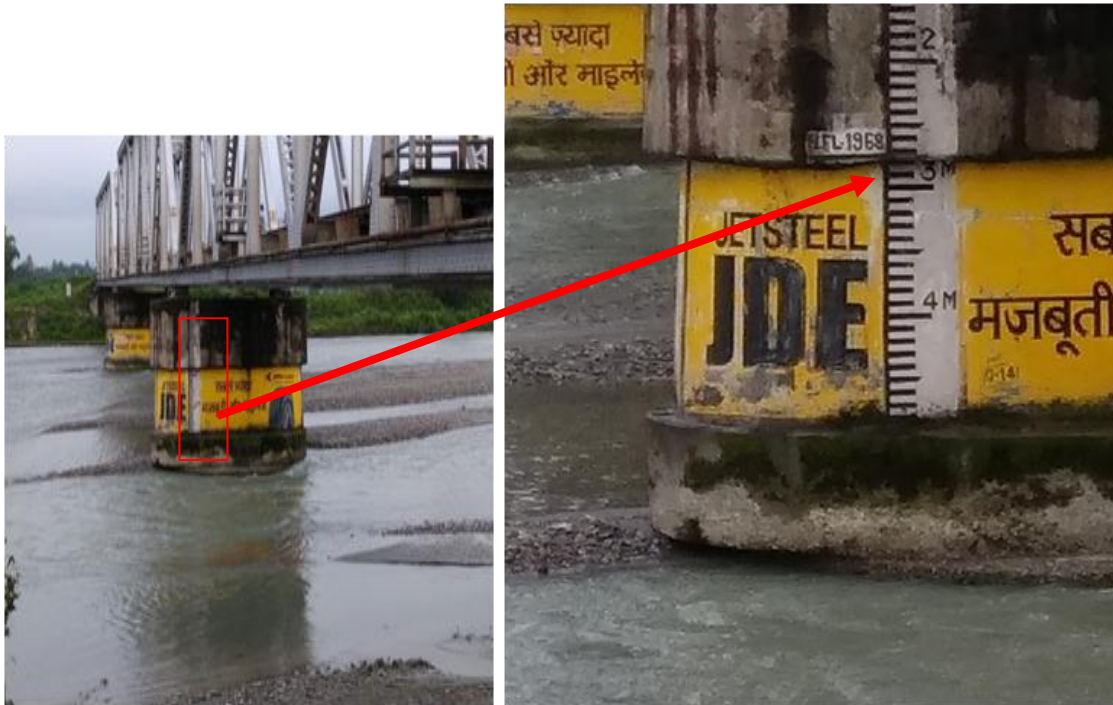
Plate 4.2.1 Field Photograph taken on 10.09.2017 displaying first railway pier from left bank over Chel River at Odlabari showing clearly CWC marked Highest Flood Level recorded during 1968.
