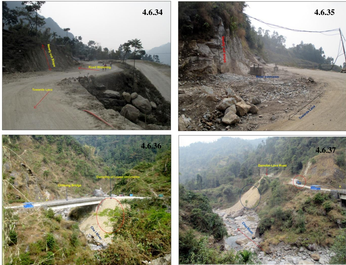
Plate 4.6.34 Road widening at near Ambhiok T.G; Plate 4.6.35 Road widening near Chitlong Bridge; Plate 4.6.36 & Plate 4.6.37 Dumping of loose sediments generated during road widening into the channel near Chitlong Bridge. A dumper/tipper truck marked with red circle can be seen returning after dumping the sediments marked with blue circle, in Plate 4.6.37.
