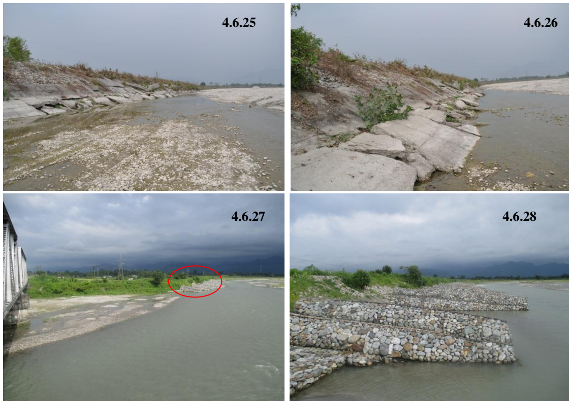
Plate 4.6.25 & 4.6.26 Damaged right embankment at transverse section C-D, (Photograph taken -21.03.2013). Plate 4.6.27 & 4.6.28 Repairing and strengthening of embankment by addition of dykes (Photograph- 10.08.2014).
