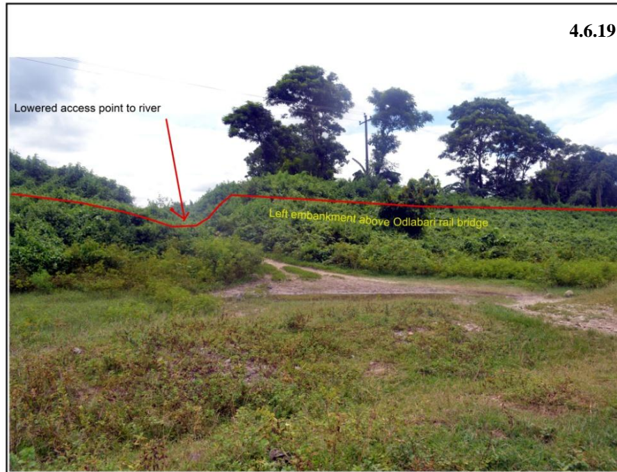
Plate 4.6.19 One of the many human breached embankment points for easy access of man and vehicles into the river.
