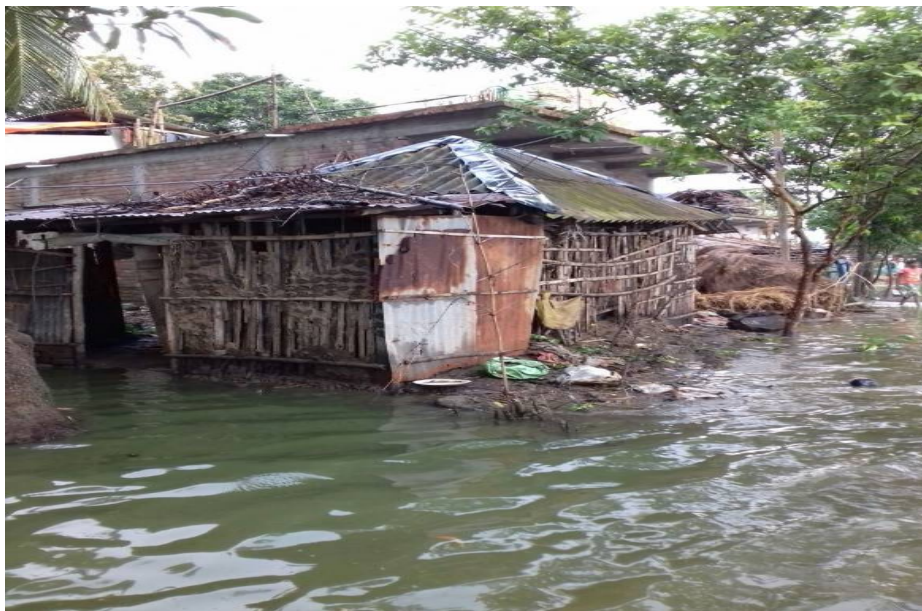
Collapsed Houses in Ghatal Flood, 2017
