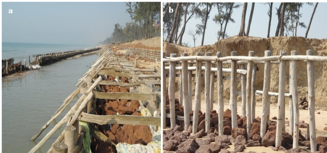
Fig. 4 : (a) landward shifting of shoreline and high tidal mark and (b) Existing damaged sea dyke of Chandpur-Jaldha sector
