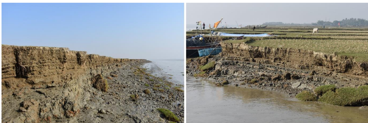
Plate 4.5: Mud-bank erosion at the right bank of Hugli river in Haldia.
